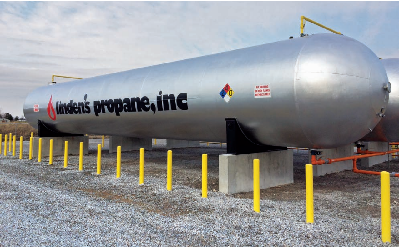
Linden's Propane has 90,000 gallons of bulk storage at its new headquarters in Wellington, Ohio, shown above, and a 1,150-gallon vertical tank and dispenser.
